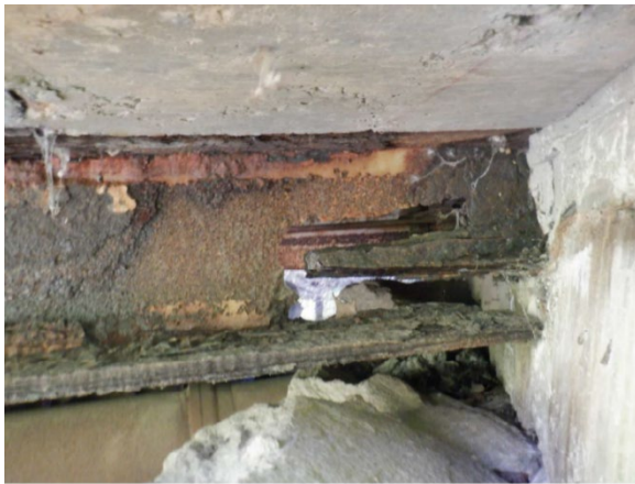
14. Upstream Steel Beam Web Rush Through Hole at Bearing
