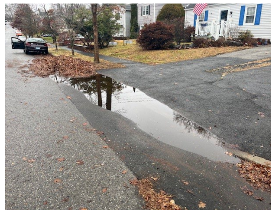
Complaint: Stormwater runoff accumulates and ponds in front of 49 Ogden Road
