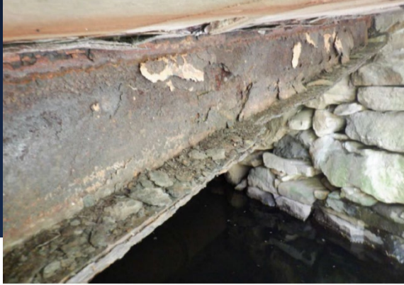
13. Upstream Steel Beam Flange Section Loss and Delamination
